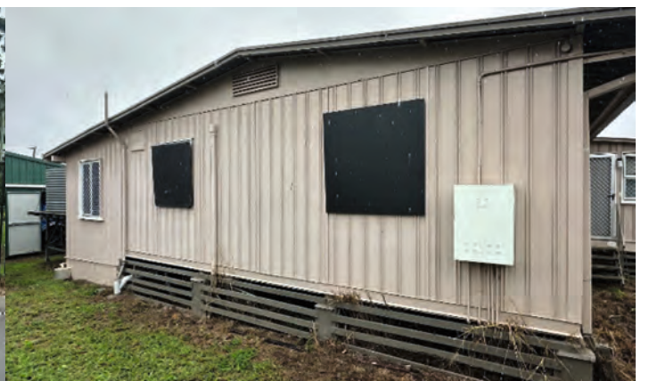
Police housing at Murgon where windows are boarded up due to offenders constantly smashing the glass.
