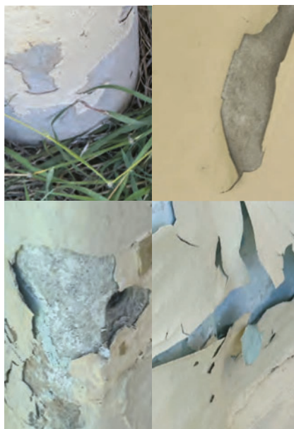
Peeling paint on police stations revealed asbestos products and exposing the asbestos to weather.
